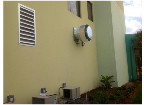
Intake and exhaust for the kitchen hood
