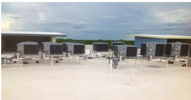
Multiple condensing units on the roof
