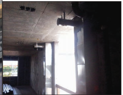
(2) metal exhaust risers with room stub-outs
