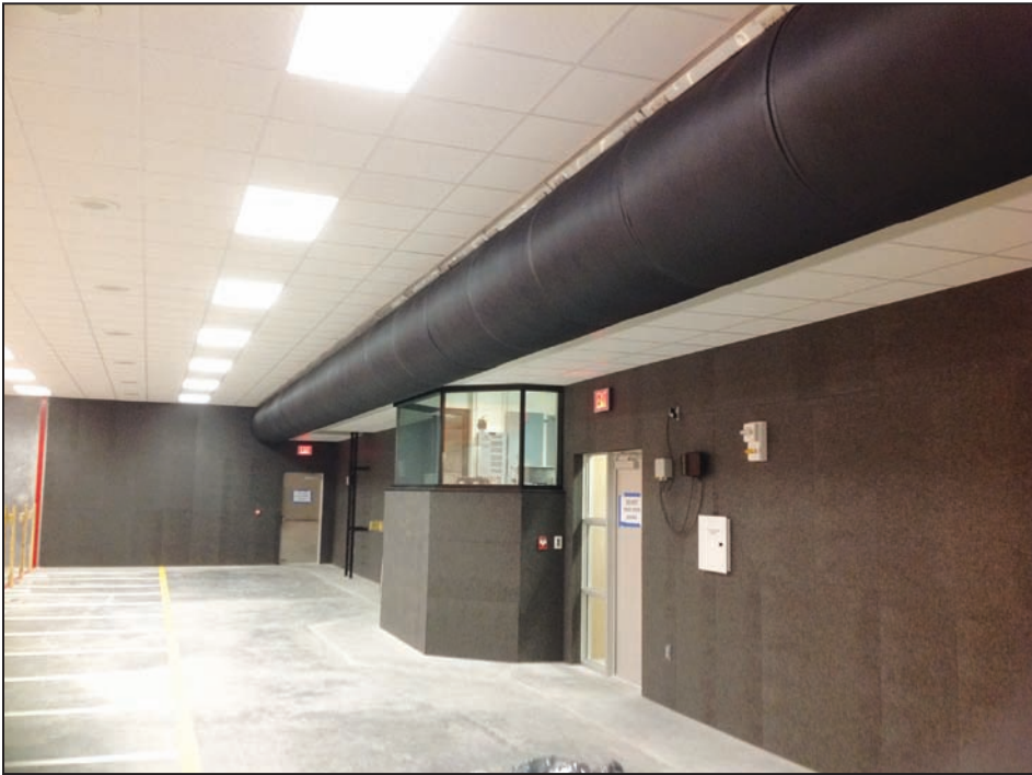
Supply Air Radial Diffuser at firing line
