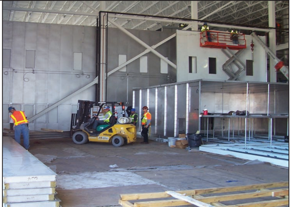
air house paint booth walls
