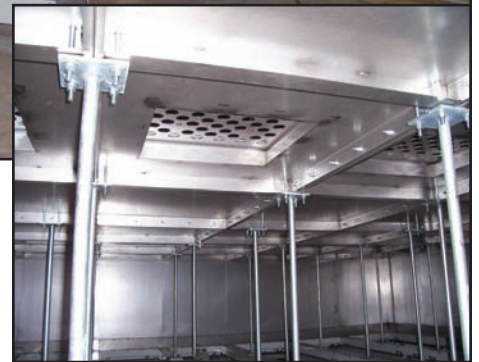
inside view of supply air plenum
