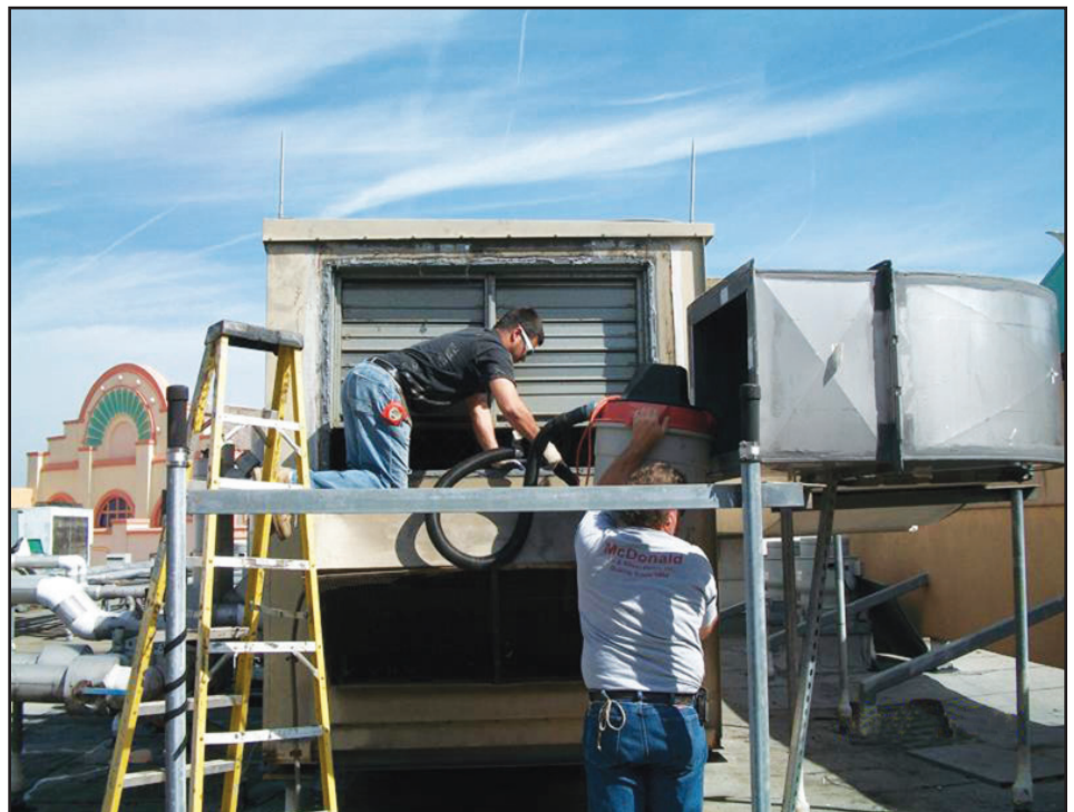
job foreman Mike Rausch Sr. and Nick Cimino cleaning and preparing for the unit tie-in
