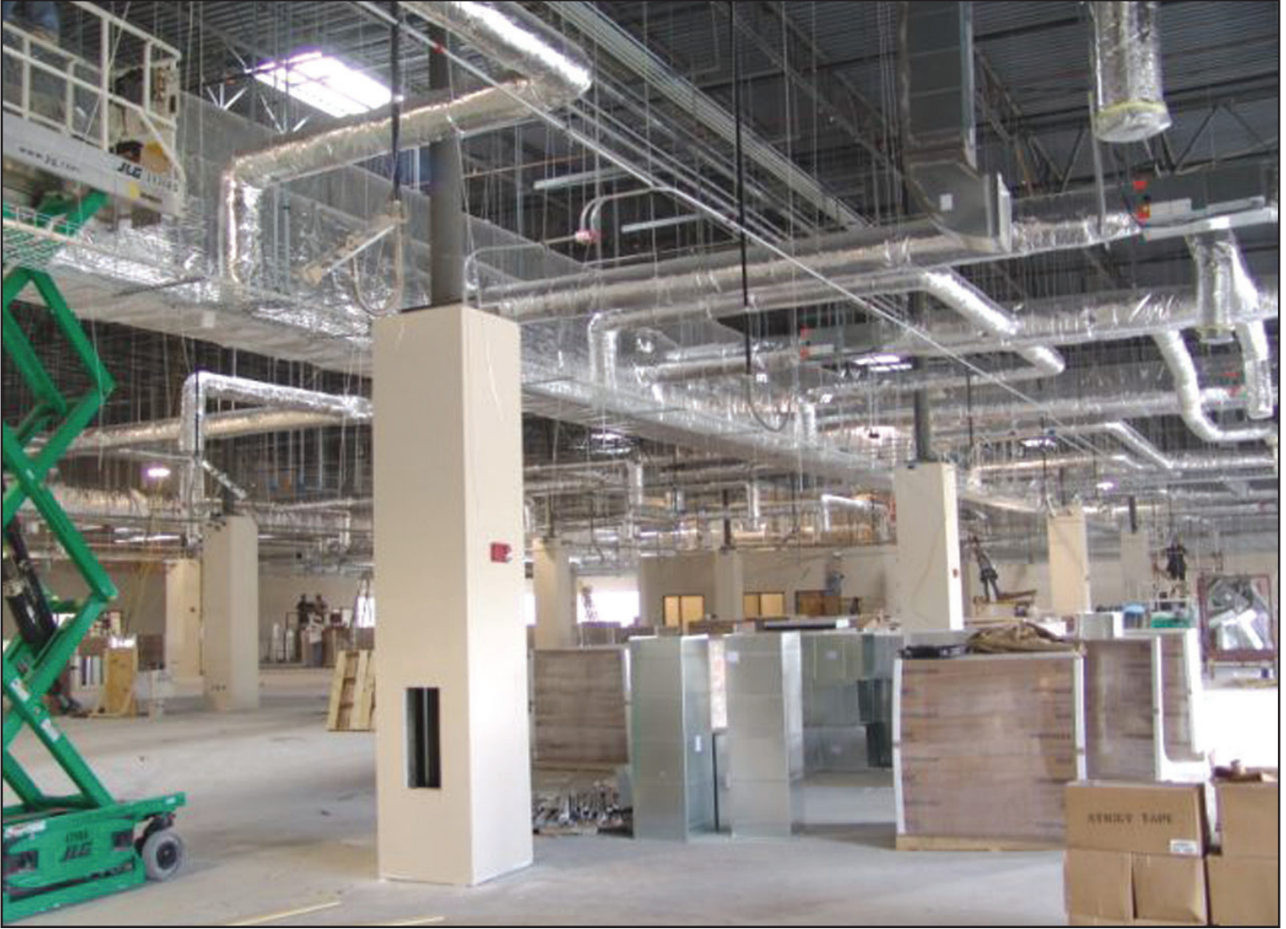
Supply duct and branches serving office space. Basic bottom of duct at 14' suspended below 23' joists. Some material is on the floor being prepared for installation.
