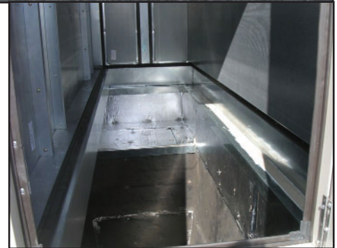
supply air opening with insulation caps
