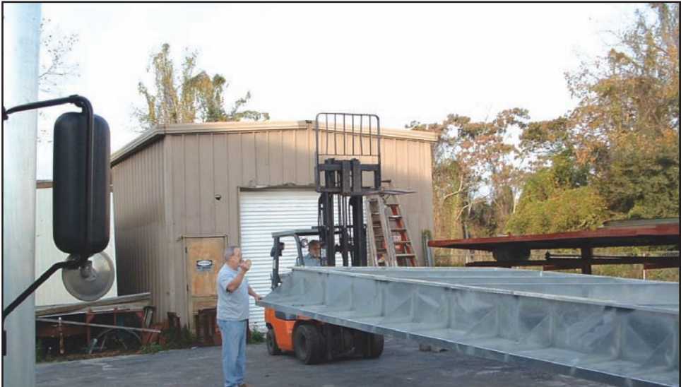
Shop Manager, Les Jones and Shop Foreman, Jim Tapan (forklift) positioning the curb adaptor in McDonald’s storage area.
