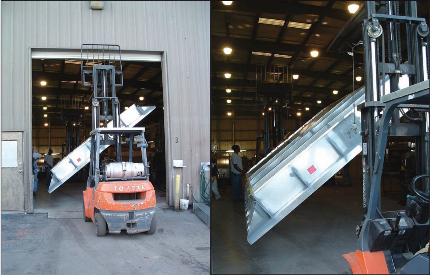
Shows the difficulty of rigging and moving the 23'-2" x 14'-4" and nearly one ton adaptor through the twelve foot wide delivery doors.
