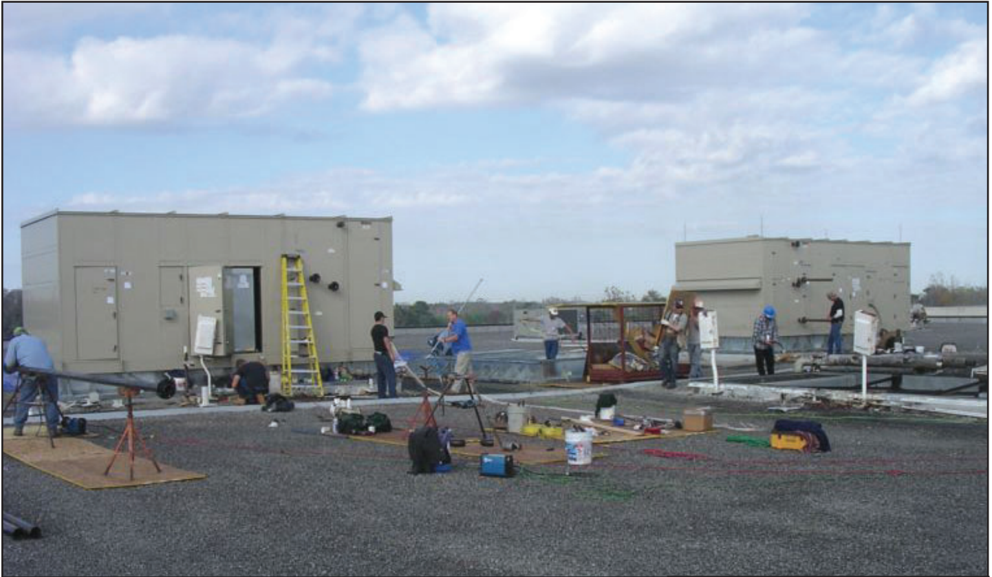
ahu 345 on right, 347 on left
