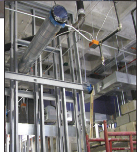
Supply air in existing area
