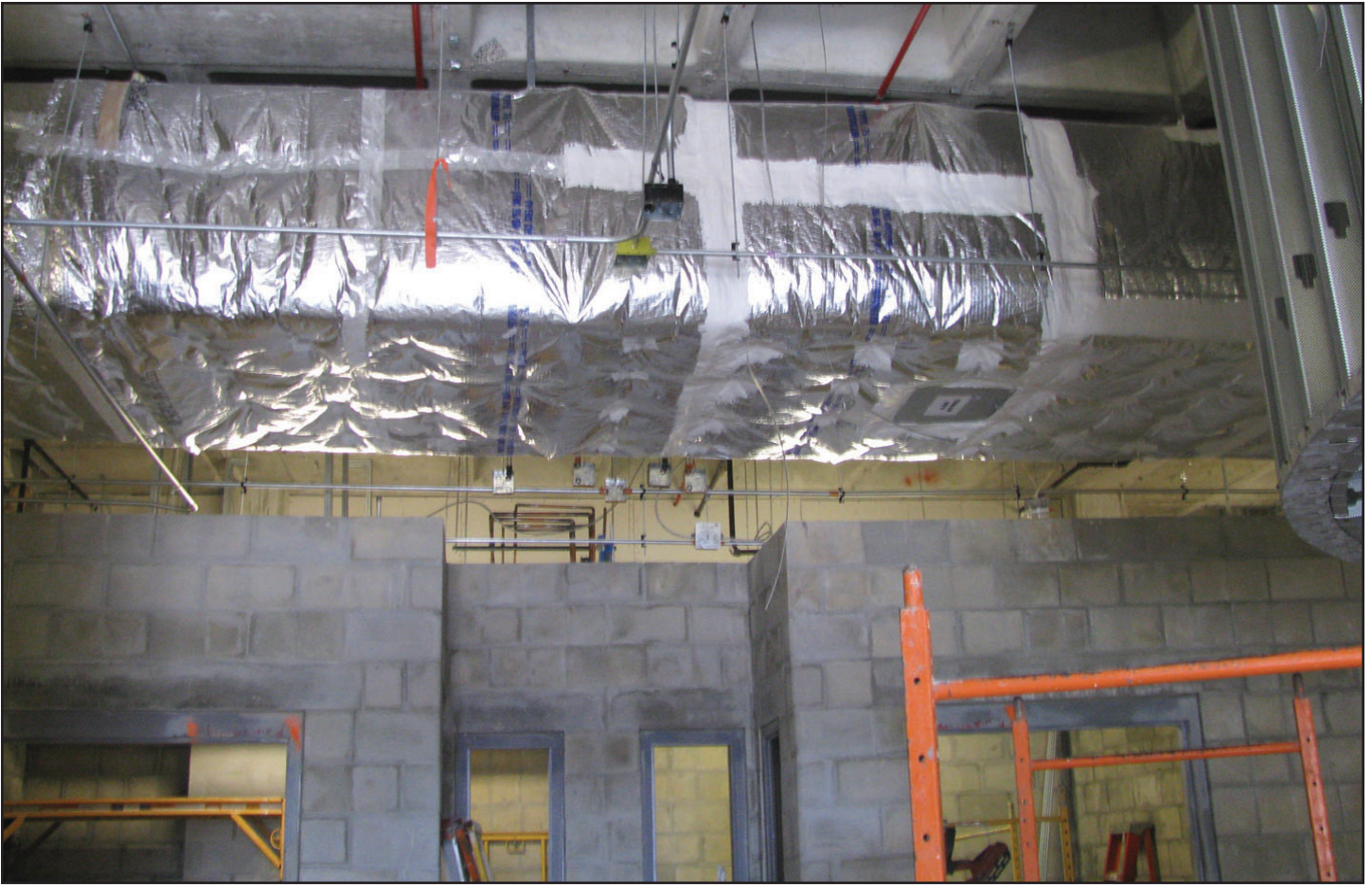
Return air ducts across psychiatric ward
