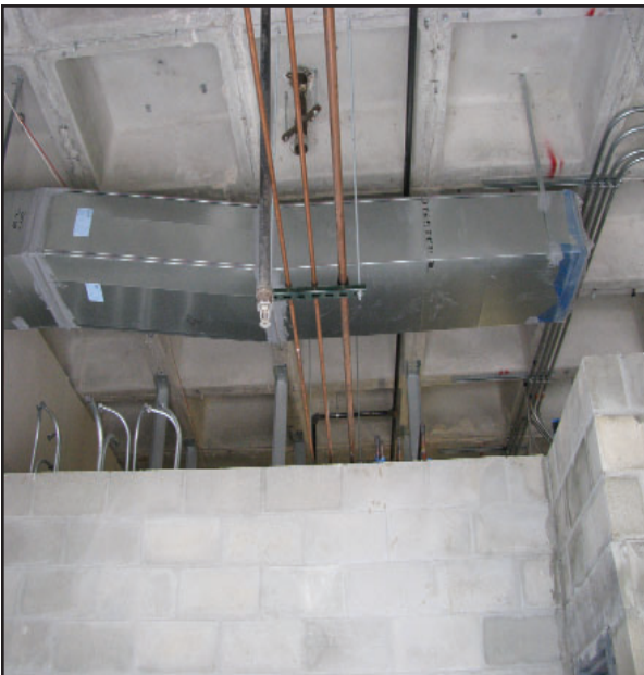
Supply air duct over psychiatric ward installed around existing pipes
