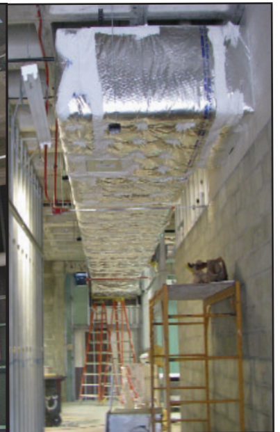
New return air duct above old emergency room
