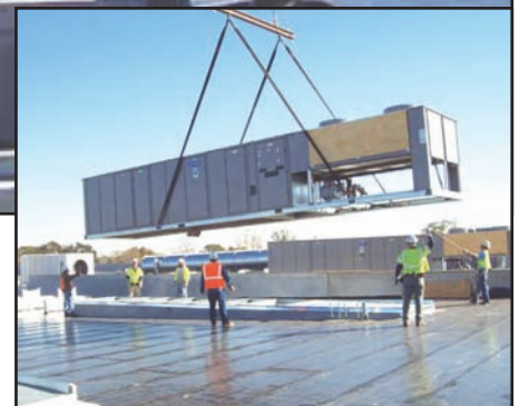
SETTING MAKE UP AIR UNIT
