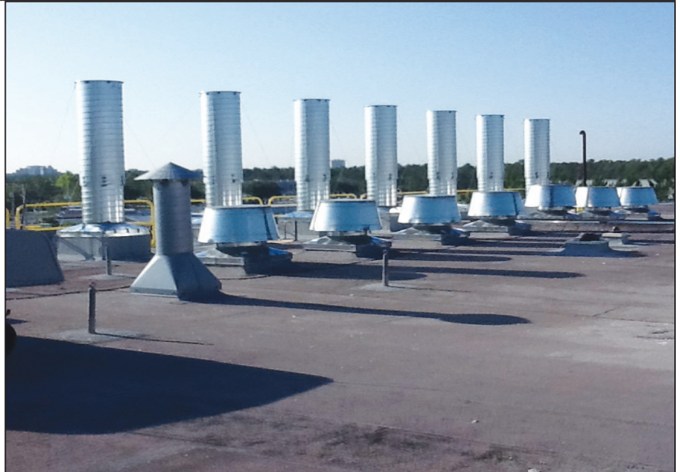
Intake stacks and exhaust stacks on roof
