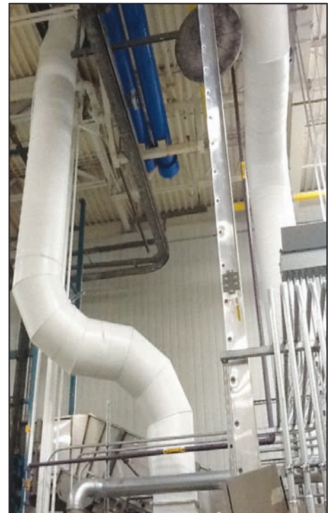
Lint collector ducts
