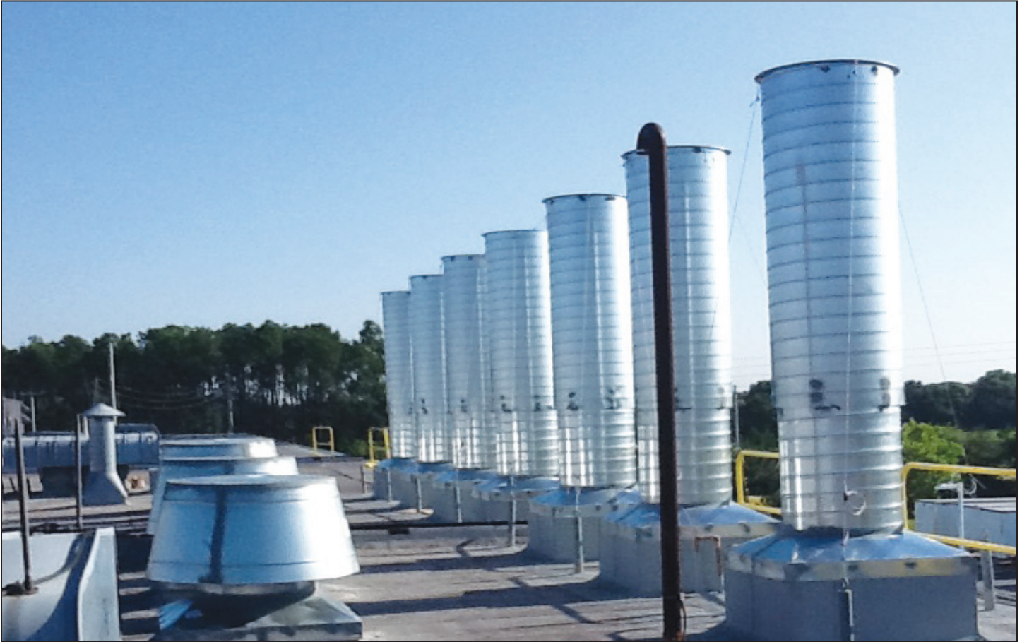
Intake stacks and exhaust stacks on roof
