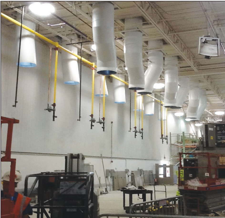
Underneath the roof showing duct drops prior to the equipment being set
