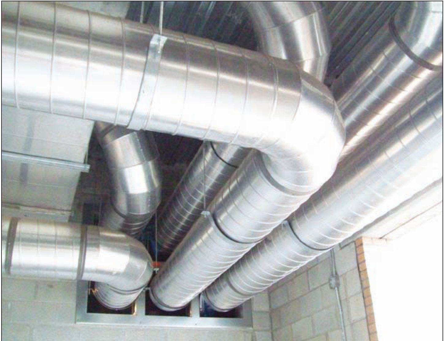
cluster of duct penetrating wall
