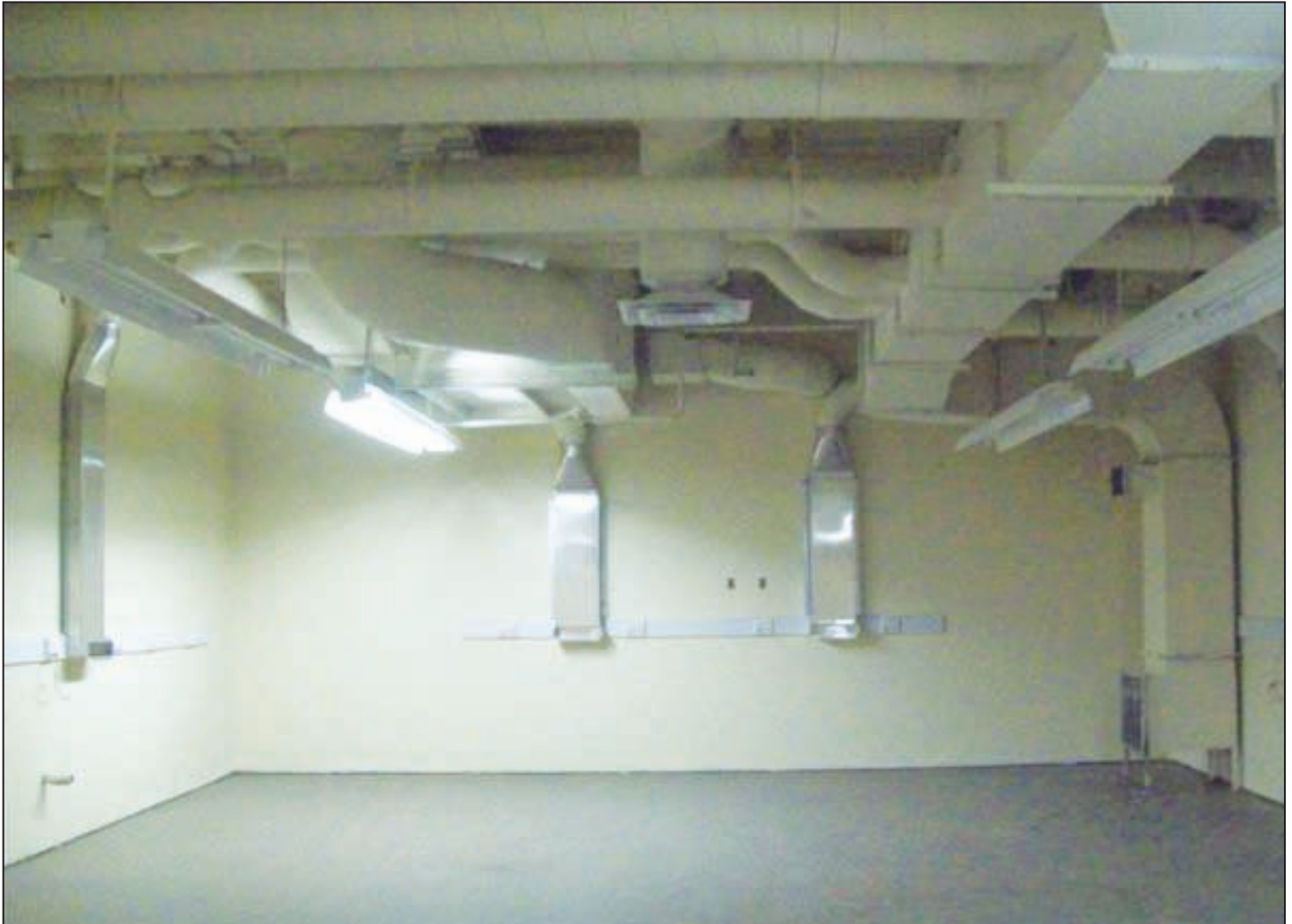
exhaust drops down to lab benches (not installed) - Aviation Maintenance Science Lab Weld Shop
