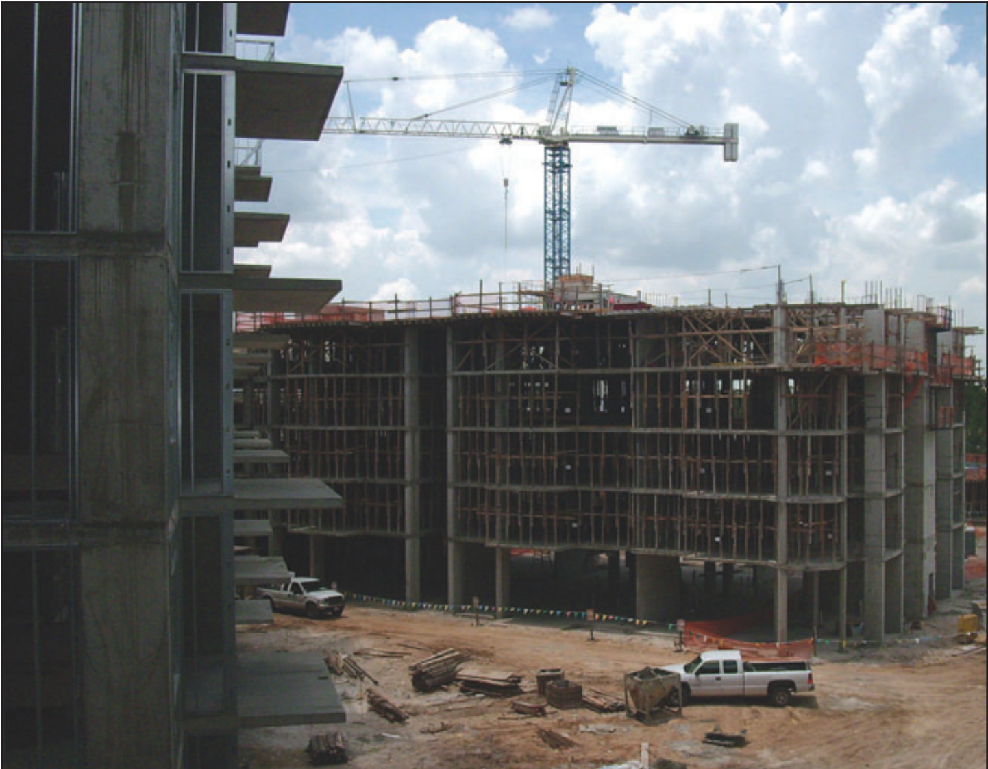
Photo shows one of the wings built to the sixth level with the tower crane shown in the back of the picture.
