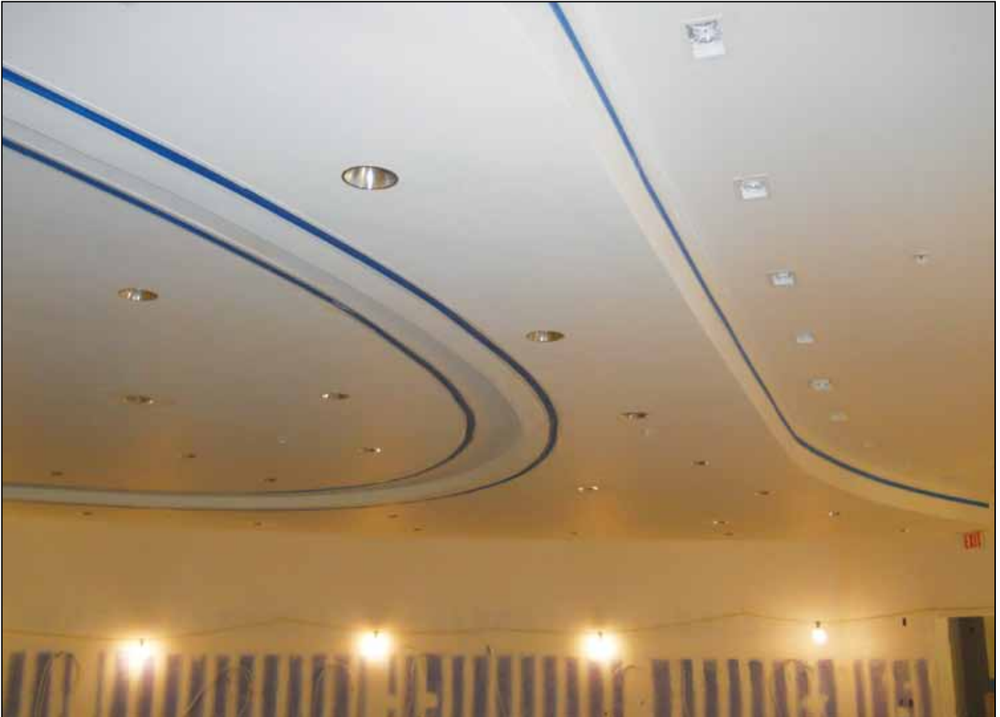
The player's locker room has custom curved linear diffusers to give the ceiling a high profile look.
